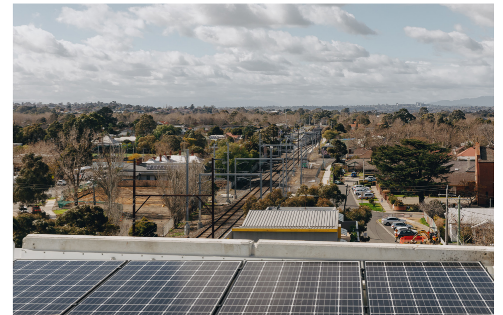
Rooftop solar. Photography by Jake Roden
