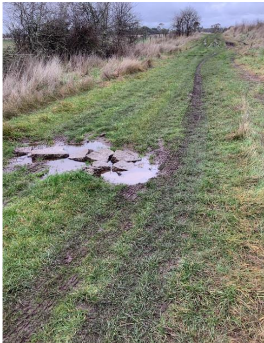
Figure 6 – Typical Potholes and drainage issue
