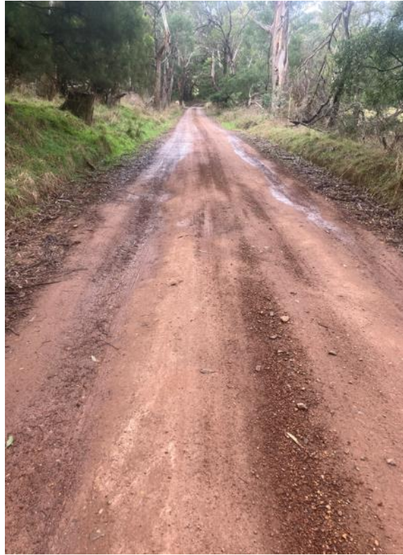
Figure 4 – Existing drainage system on Segment 2
