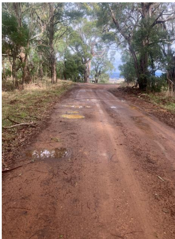
Figure 8 – Existing potholes on segment 2.
