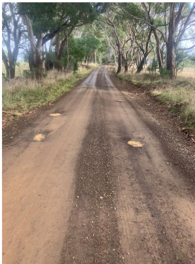
Figure 7 – Existing potholes in Segment 1
