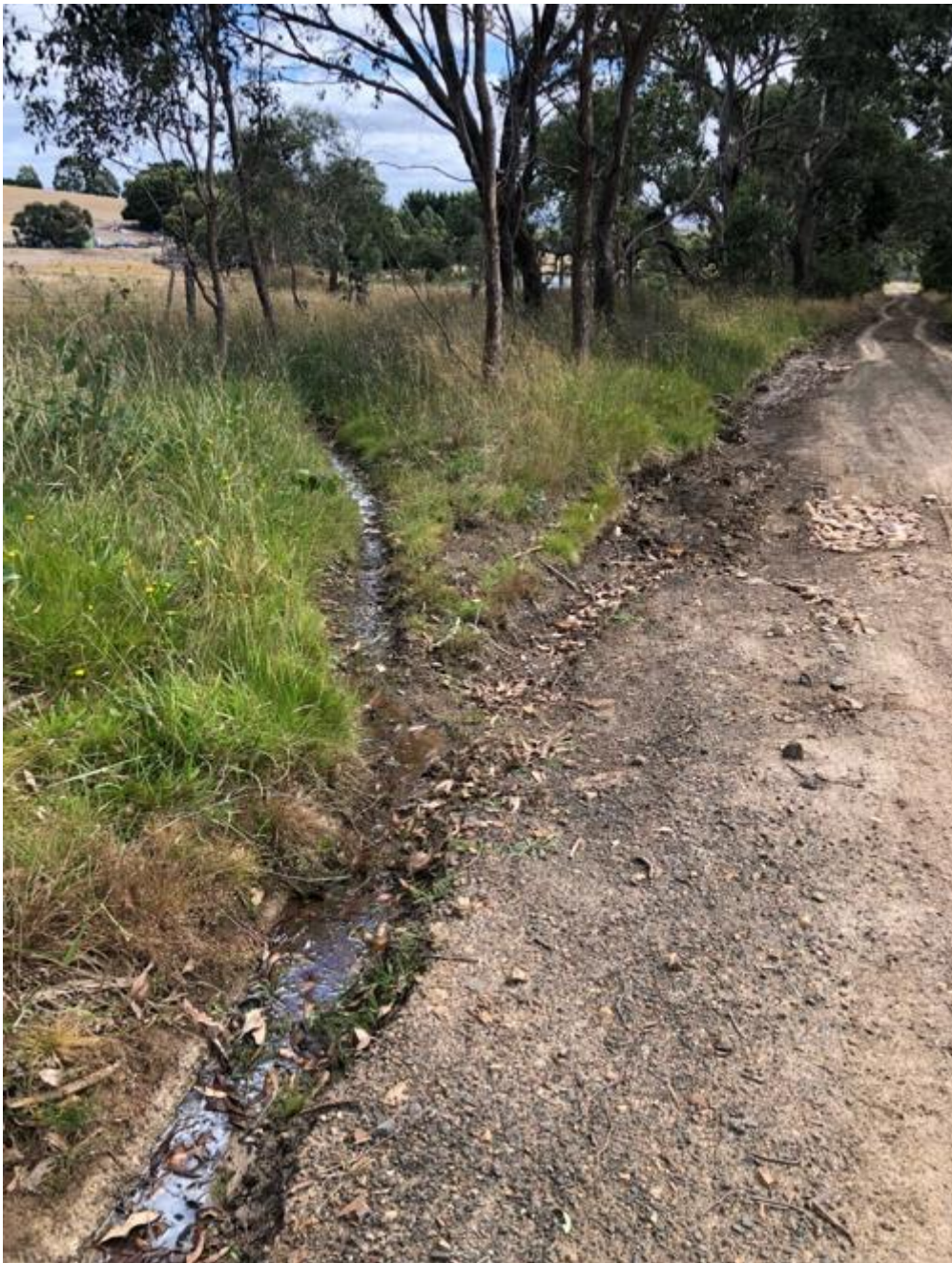
Figure 7 – Existing drainage system
