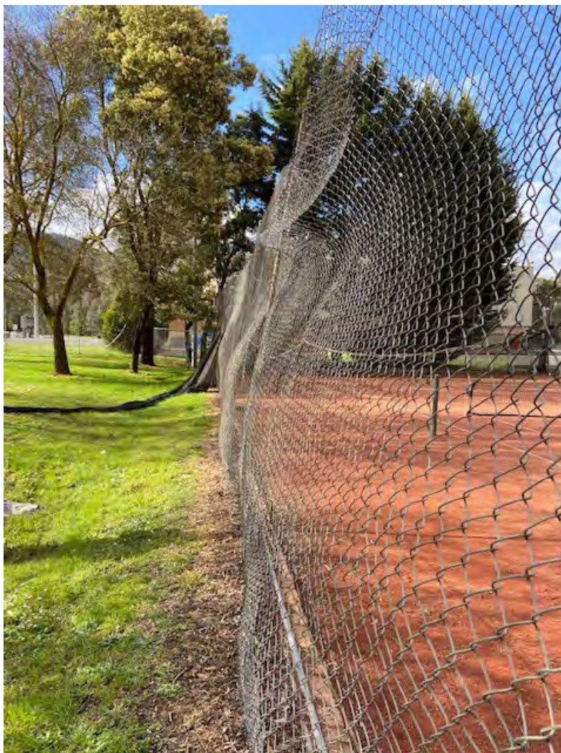
■ Court 1- Bulging fence, bent posts, no top rail. (2023).
