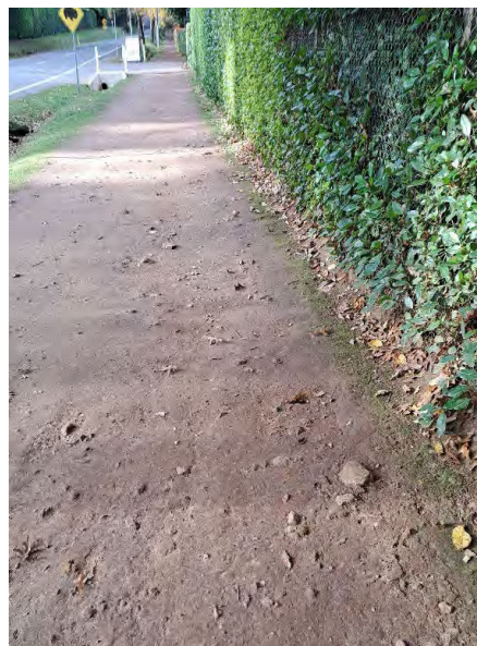
This a picture of the road reserve in front of Durrol next door to Forest Glade. This area always has green grass and mosses, it has been totally destroyed, like many locations on Mount Macedon
