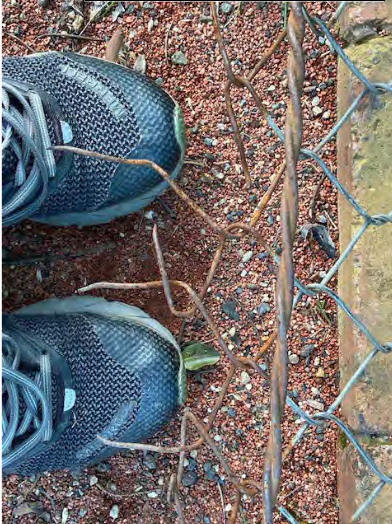
■ Courts 1-4. Frayed wire (2023).
