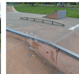
Cracking / rough surfacing on obstacles.
