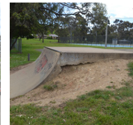
Erosion of earthworks around skatepark.
