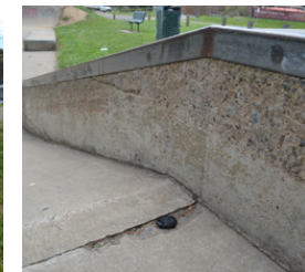
Cracking / surface damage at joints.
