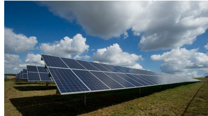
Victoria's biggest solar farm under construction amid debate over lost agricultural land - ABC News
