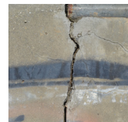
Concrete cracking at joints.
