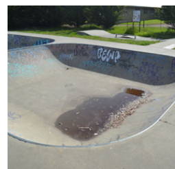
Pooling of water at base of bowl.
