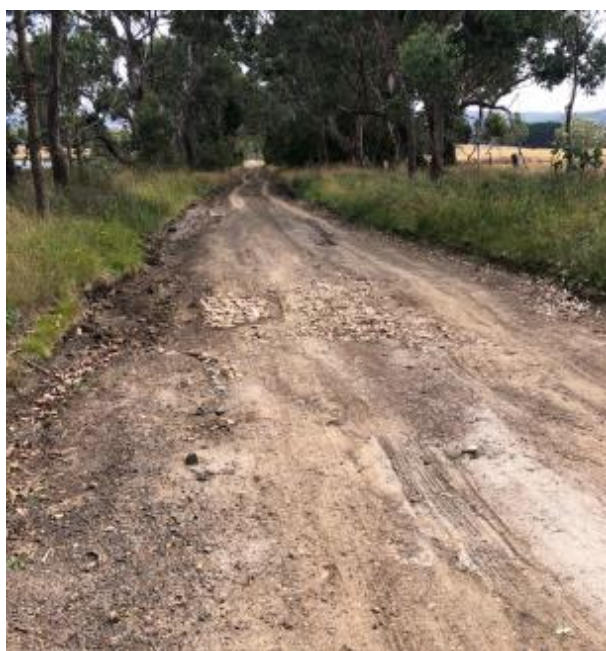
Figure 6 – Typical Potholes and drainage issue
