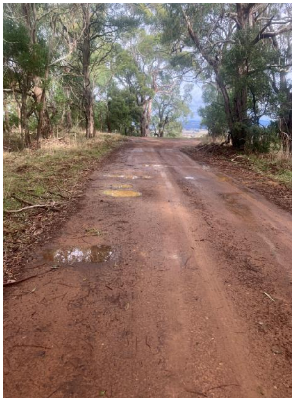
Figure 8 – Existing potholes on segment 2.
