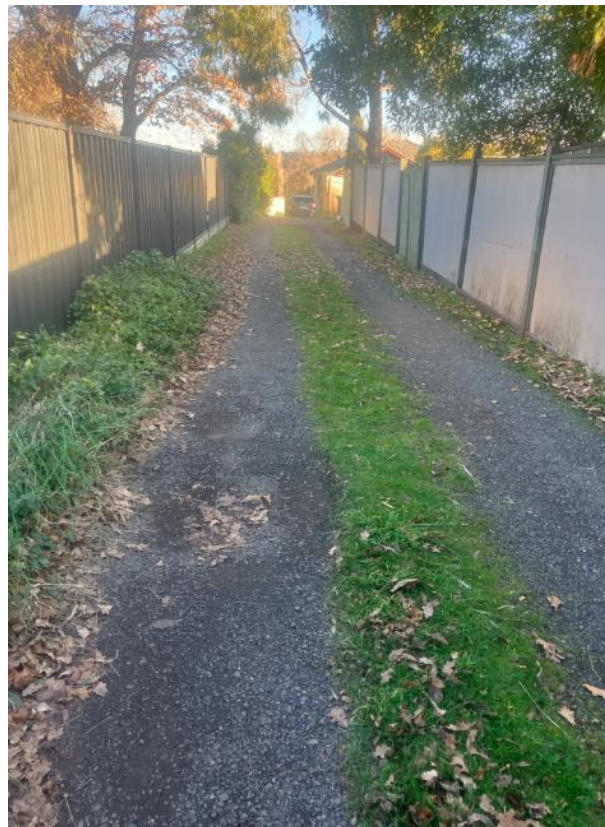
Figure 7 – Lack of drainage system
