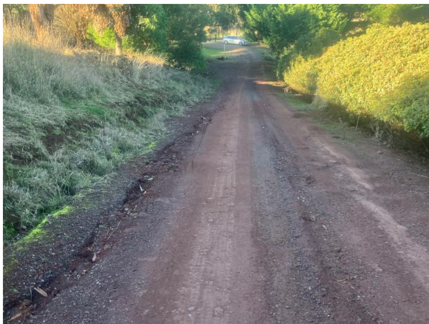
Figure 8 – Scouring of the road surface along the longitudinal section
