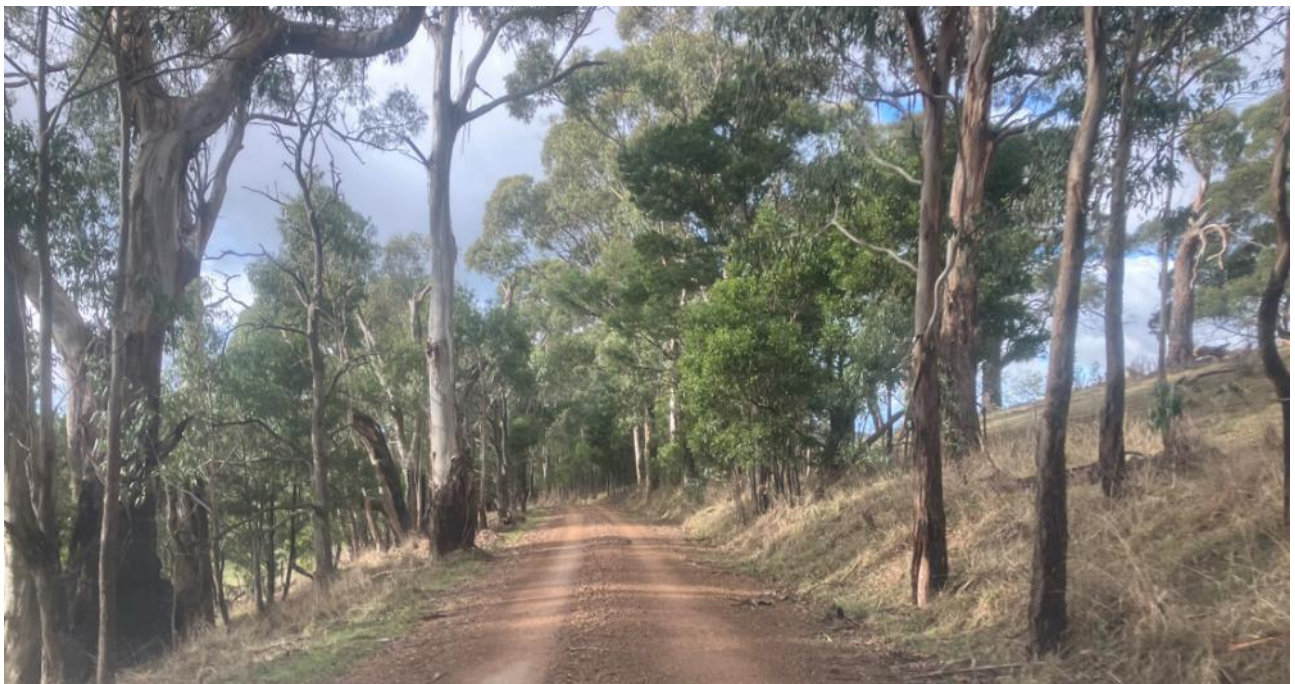
Figure 5 – Existing drainage condition on Segment 3.
