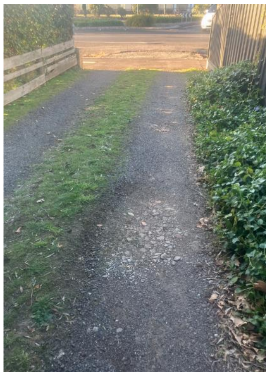
Figure 8 – Several potholes along the road carriageway and limited sight of pedestrians and vehicular movement on High Street from Access Lane
