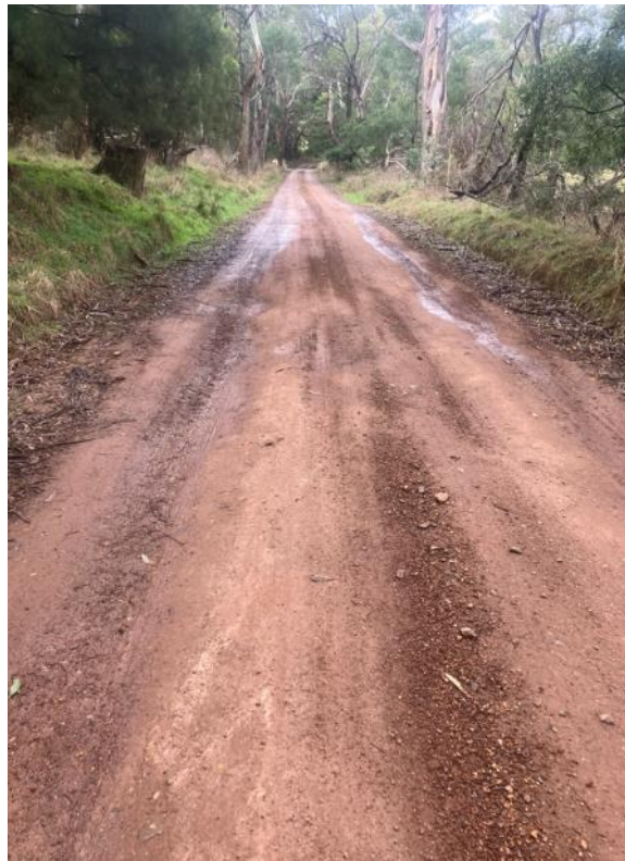
Figure 4 – Existing drainage system on Segment 2
