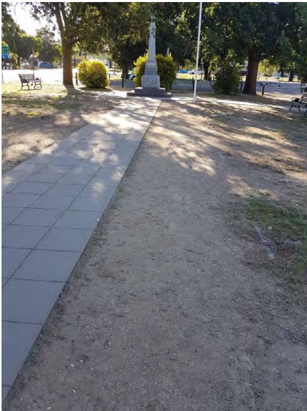
Figure 5 Further erosion and damage.
