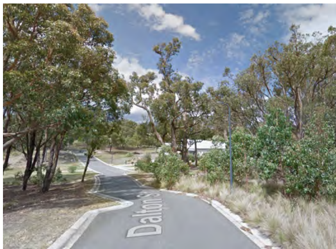
Figure 37. Example of vegetation encroaching on the road envelope
