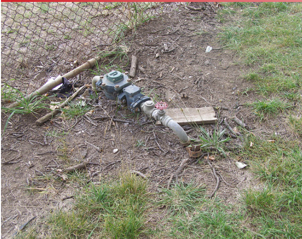
Sustainability Fund may support better use and management of the water metre, which is currently exposed.
